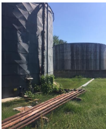
Fig 4.a. Thermal storage in existing tanks
